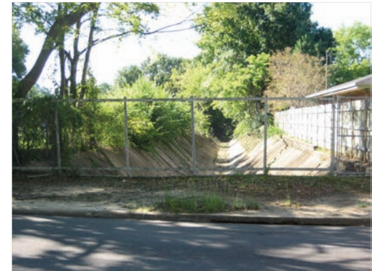
Concrete “flumes” can create hazards for neighborhood residents if not properly maintained.
