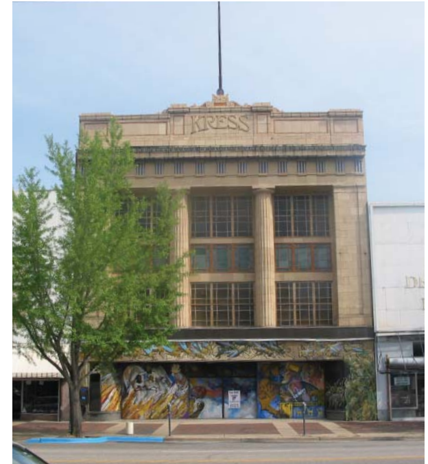
Many façades along Dexter Avenue are in need of repair.
