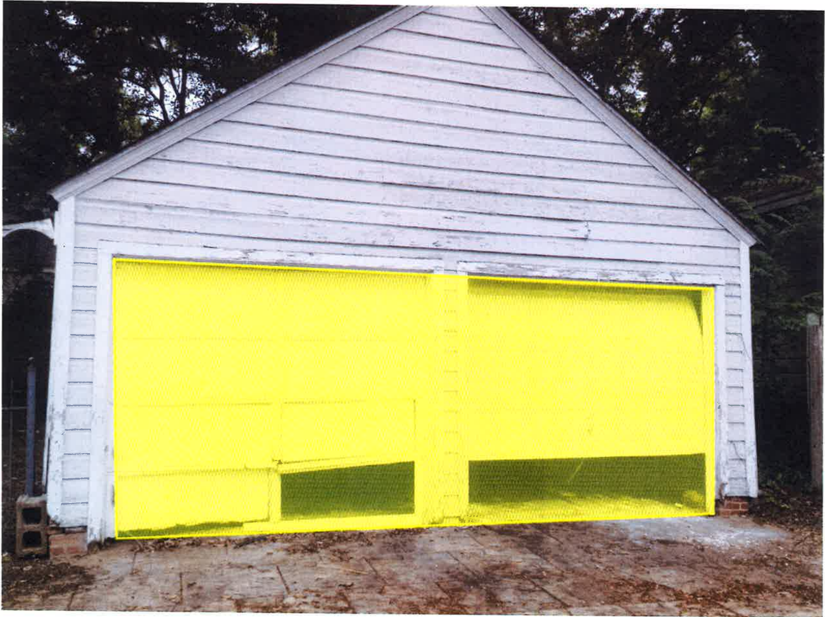
REBUILD DETACHED GARAGE EXACTLY THE SAME EXCEPT WITH A DOUBLE GARAGE DOOR
